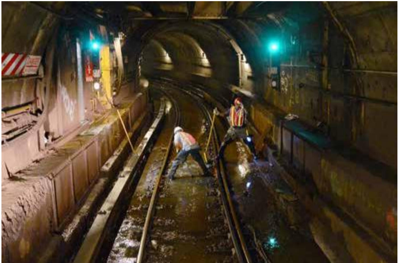
MTA workers clear a clogged drain near the Cortlandt Street subway station to prevent flooding during a heavy rain event
