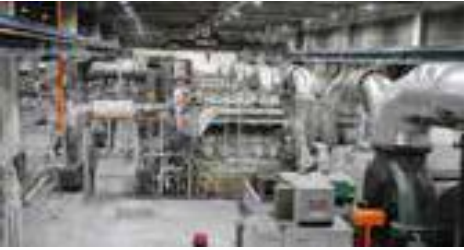
North River Wastewater Treatment Plant Combined Heat and Power Facility
