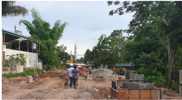
The workers on the construction site have not yet fully complied with labor protection;
