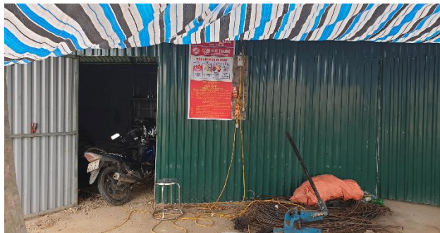
Not equipped with fire extinguishers in camps and material warehouses
