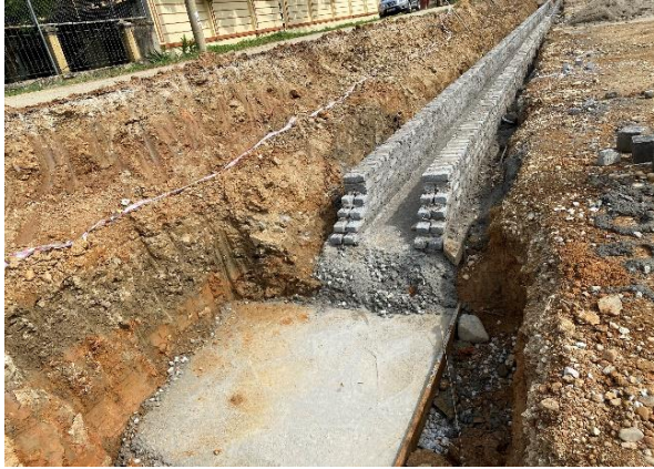
Tay Minh Khai Road: There is no construction solution to ensure absolute safety for the high difference positions between people's houses and the ground.
