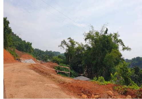
Key and dangerous location has been warning by contractor (Nam Cut bridge item)
