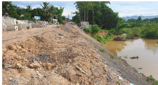
There are no isolation barriers for households that have not been relocated, living in the construction area, as well as separating existing construction sites and residential areas.
